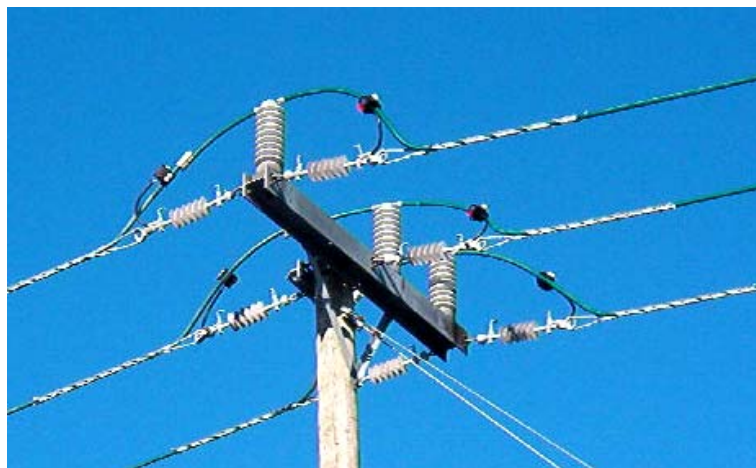
Fig.6. Straining of insulated conductor ( 24 kV, top of angle-strain pillar )
