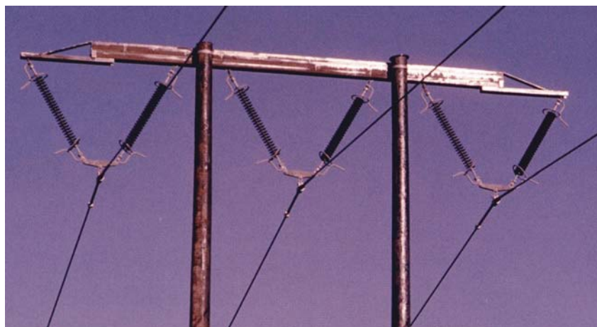
Fig. 2. Overhead line with insulated conductors ( Norway, 145 kV )
