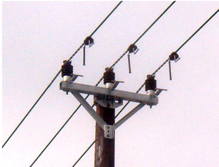
Fig. 5. Fixing of insulated conductor to supporting insulator ( 24 kV, top of supporting pillar ).
